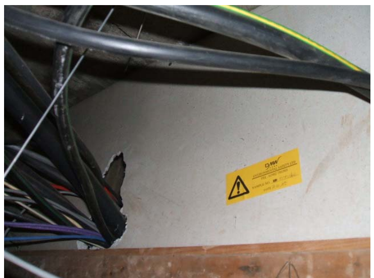
Damaged Fire Stopping spotted on a DMW Survey. This is dangerous from two standpoints, at least!
