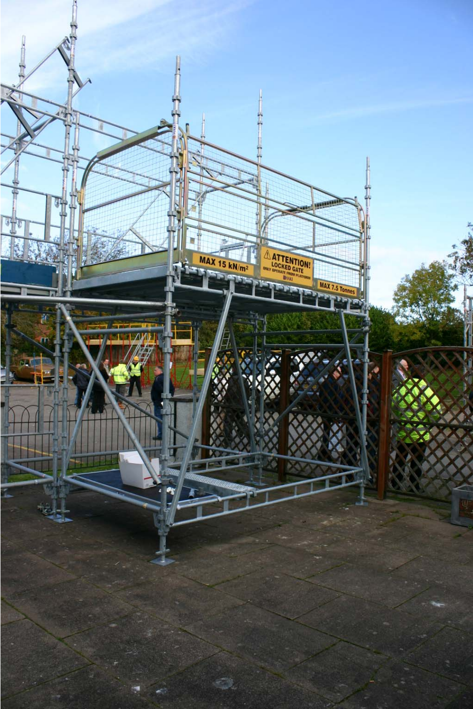
The HAKI Loading Deck security gate
