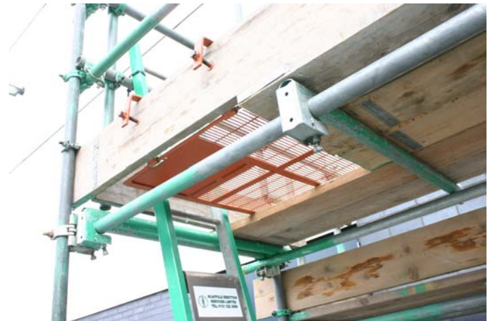
The SES Scaffold Access trap.
