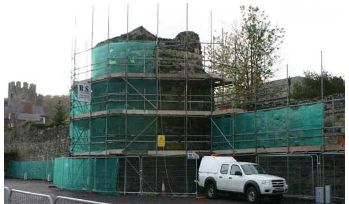
1 Working Lift but 3 lifts actually boarded
