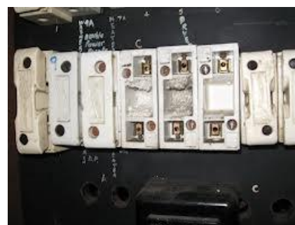
Electrical Equipment Arc Shields, ACM in fuses and electrical contacts
